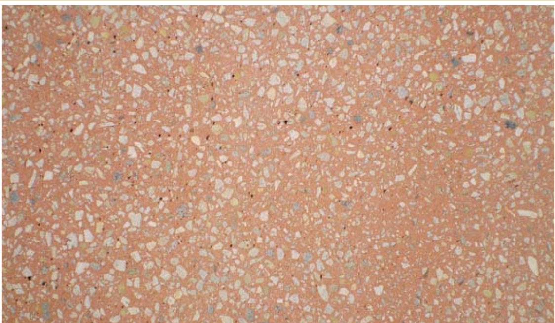
All holes and imperfections which appear after grinding can be filled with a special grout mix.
